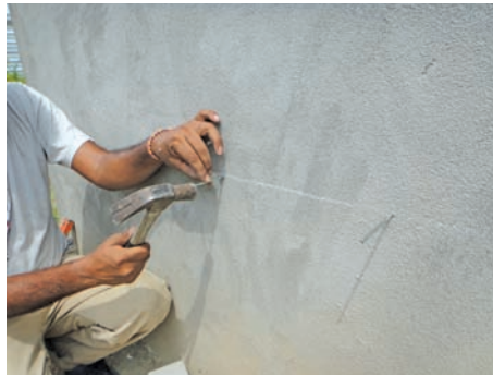
b) Hammer concrete nail to cement wall after cleaning & roughening the wall.
