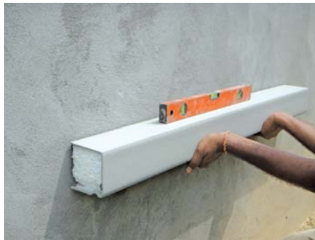
e) Push the foamcrete cornice to wall which has already nailed, roughened & cleaned.
